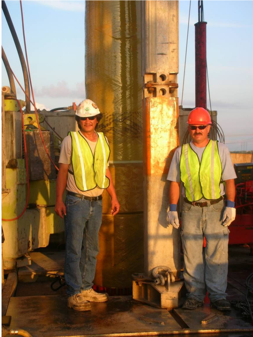
Shown above: FPI installation crew from the Houston factory on the Youngquist Brothers Drilling rig. Dan Troung (L) and Jose Tapia (R)
